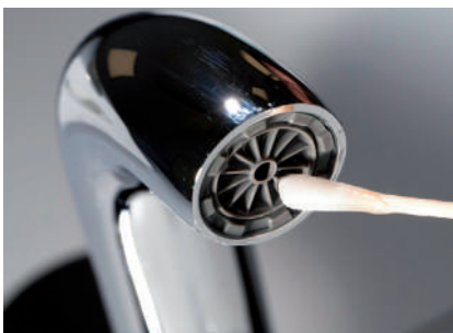
Figure 5.2: Swabbing the Inside Surface of the Tap Outlet or Flow Straightener
